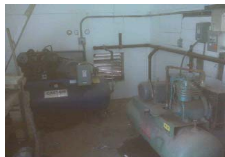
Compressors in Compressor Room
