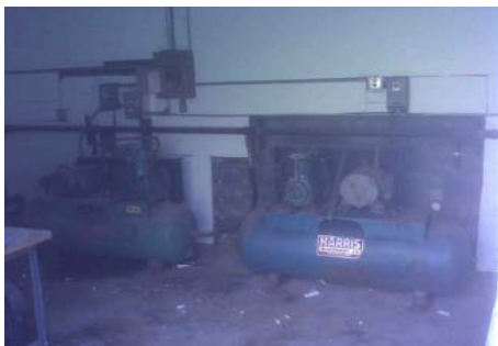
Compressor Room on East Side of N. Building
