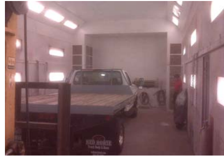
North Bldg - Large Spray Booth
